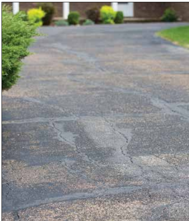
Surface cracks in a driveway may indicate a problem that requires immediate attention.
