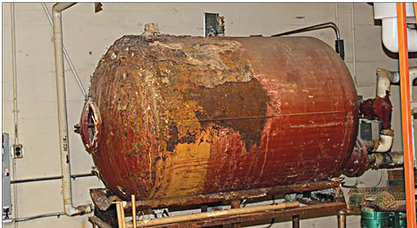
The plan include replacing end-of-life boilers from 1984 with an energy-efficient model.
